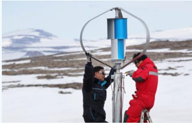
300W turbine installed at the South Pole for scientific research project
